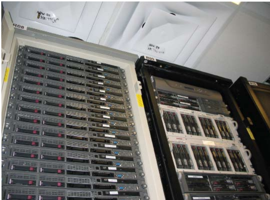
Two of the six server racks in the Bush Science Center server room. Two of the four ceiling diffusers from AHU-3 are visible above.
