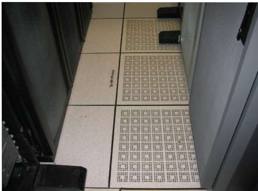
Eight raised-floor diffuser tiles provide 3,360 cfm; ceiling-diffuser design airflow is 850 cfm. Nominal design server heat load is 48 kw, with 54°F supply air, 74°F average space air, and 90°F hot-aisle exhaust.
