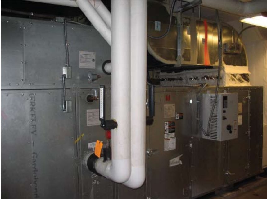
Airflow in AHU-3, a modular air-handling unit, moves from right to left. The chilled-water coil module is directly beneath the hot-water coil module in a blow-thru hot-deck/cold-deck arrangement. The mixing-damper modules are on the left.
