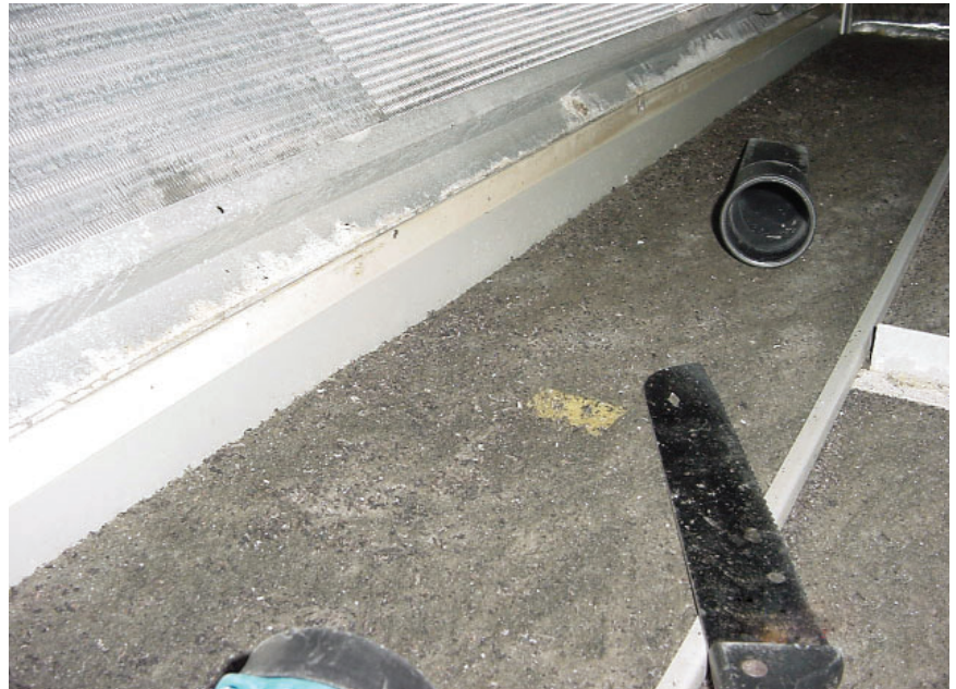
PHOTO B. Granular particulates shed from an air-handler coil.
