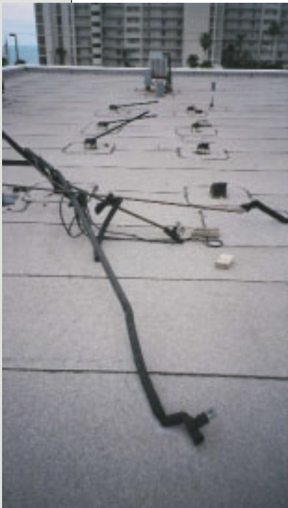
Remnants of piping and support brackets where solar hot-water panels were destroyed by Hurricane Francis in September 2004. The panels damaged the roof deck and one of the condenser coils as they were blown across the roof.
